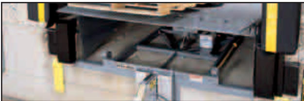
Unsealed leveler pit.
