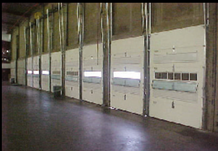
Multiple Universal GX-4000 doors with three Universal Ventilation panels at a sugar processing plant.
