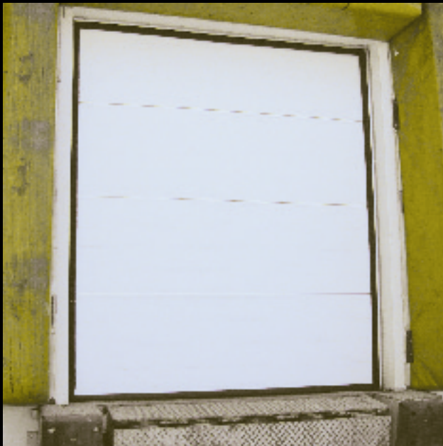
Complete Universal GX-4000 door at a food processing facility.
