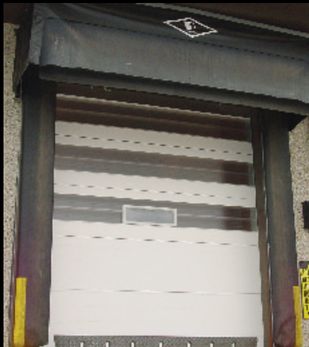
A Universal GX-4000 door with Day-Lite Translucent slats and a window at a manufacturing plant.
