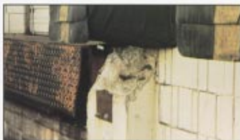
Bumper failure causes costly concrete repair, damage to dock equipment and building damage.
