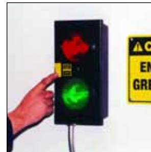
VBR-300 M inside lights.
